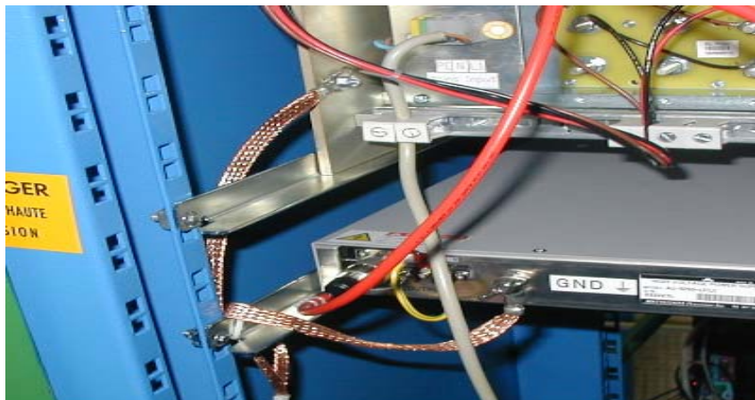
LV power supply grounding (top) HV primary power supply grounding (bottom)
