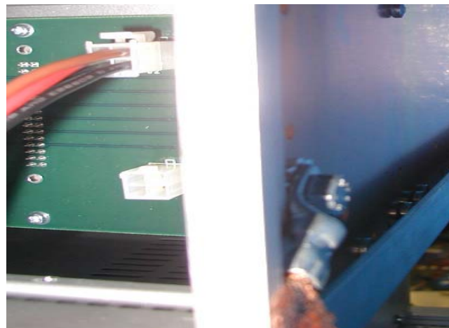
HV crates grounding point
