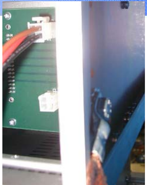
HV crates grounding point
