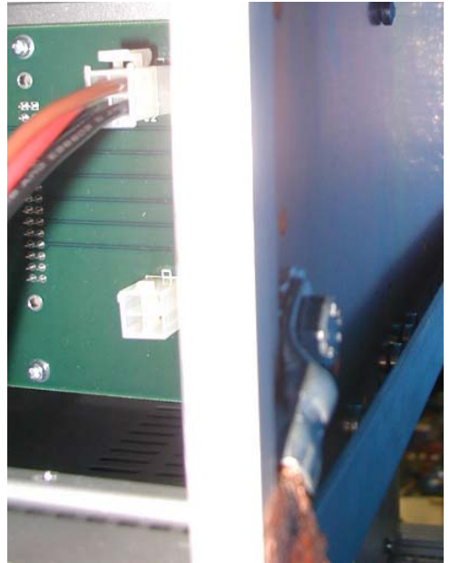
HV crates grounding point
