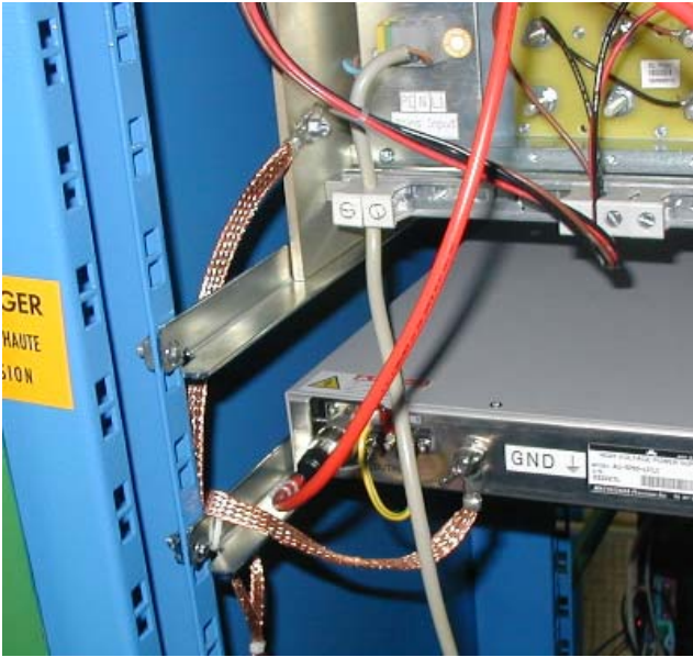
LV power supply grounding (top) HV primary power supply grounding (bottom)
